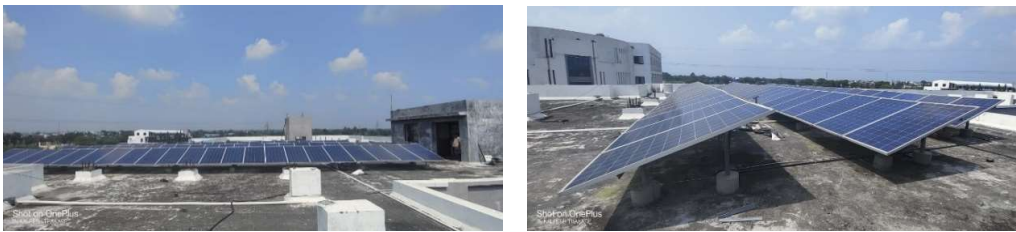
Roof Top Solar Panels and Inverters
