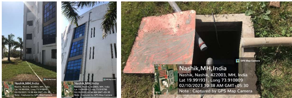
Rain Water Harvesting system
