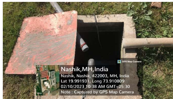
Rain water Harvesting system and recharge pit
